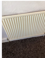
Ref # 11.7 - Gas central heating
