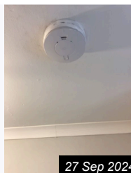
Ref # 4.1 - Smoke Alarm in hallway
