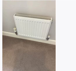
Ref # 12.7 - Gas central heating
