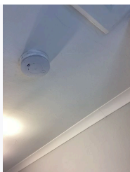
Ref # 4.1 - Smoke alarm on landing
